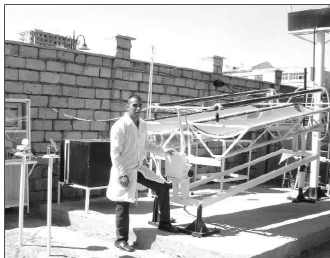
Figure 1. Solar plant with parabolic trough concentrator
