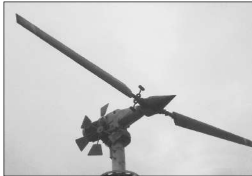
Figure 3. The general view of wind plant
